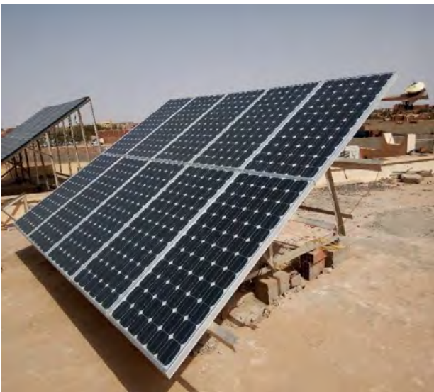
Fig. 1. The 1.75 kW of PV array installed in the roof of URERMS, Adrar.
