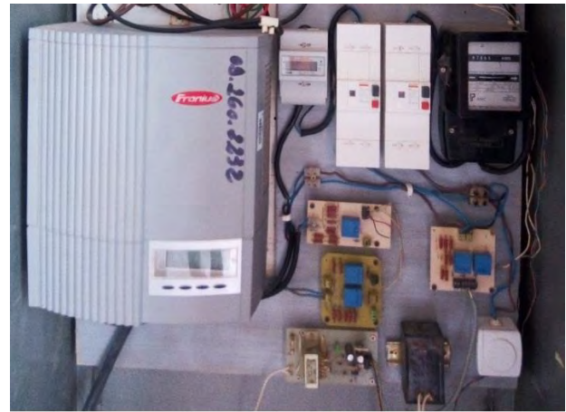
Fig. 2. View of PV Inverter, conditioning circuits, electric meters and circuit breakers
